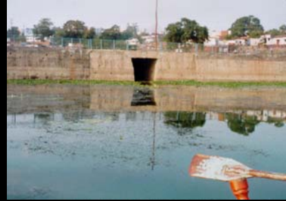
Outfall near VanVihar
